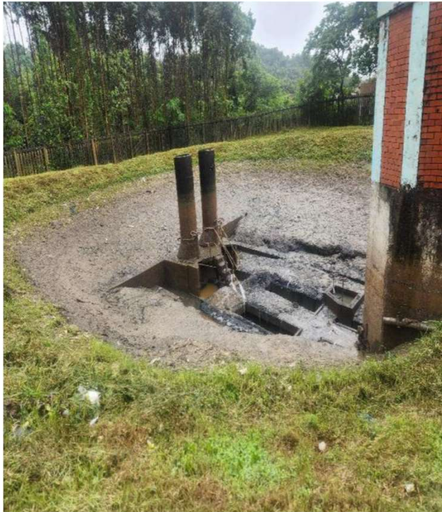
Sewage holding area at the inlet of the pump station – posing a risk to groundwater sources and nearby households.
