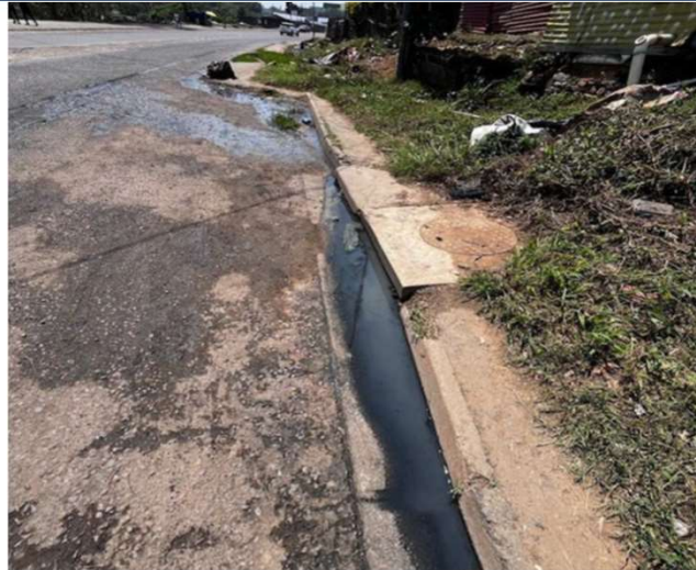
Sewer overflows and blocked drainage along the roadway and pavement.
