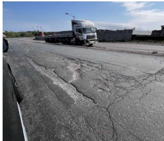
Pavement distress evident: surface rutting, delamination, transverse cracking, and uneven surfacing
